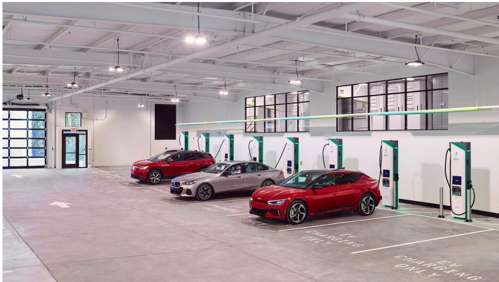
Figure 7.3.1 EVs getting charged in an enclosed EVCS
